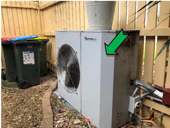
Photo 9. Exterior, backyard, air conditioning unit – non ODS depleting R410A refrigerant.
