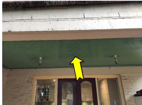
Photo 4. Exterior, backyard, eaves – suspected lead-containing green upper coloured paint system.
