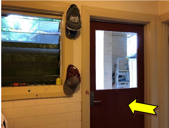
Photo 7. Interior, throughout, door – suspected lead-containing red upper paint system.
