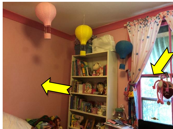
Photo 6. Interior, girl's room, walls and window frames – suspected lead-containing light and dark pink upper coloured paint systems.
