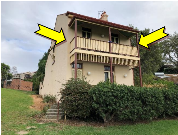
Photo 3. Exterior, throughout, walls and features – suspected lead-containing cream and red upper coloured paint systems.
