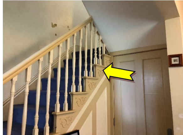
Photo 8. Interior, throughout, staircase – suspected lead-containing beige coloured paint systems.
