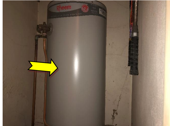
Photo 2. Interior, cupboard, hot water heater – suspected SMF internal insulation material.
